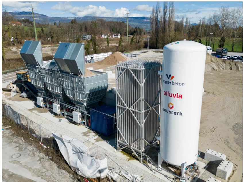
CO 2 storage facility in Biberist (CH).
